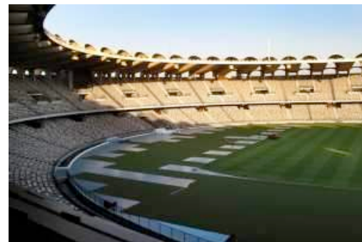
Workers renovate the pitch at Zayed Sports City. The pitch was tested at the game between Manchester City and the UAE last month. Delores Johnson / The National
